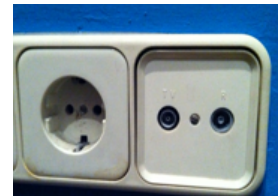
An antenna plug next to a power point
